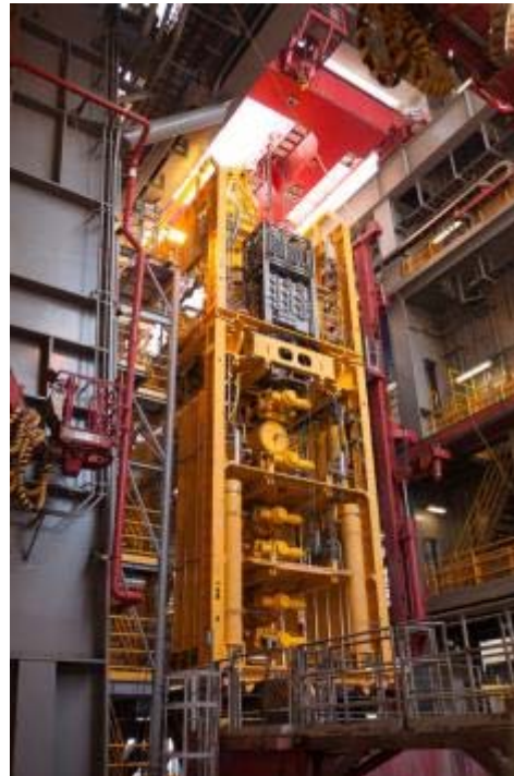
Blowout Preventer (BOP)
